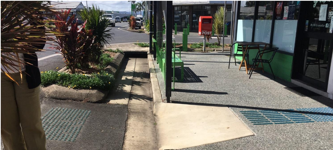
Figure B3: Height of road and drains relative to floor level of building
