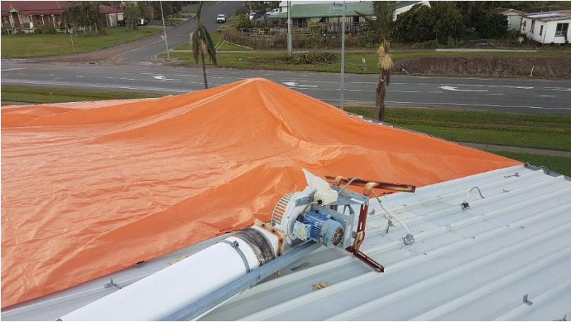
Figure B1: Failed roof vent and damage to interior
