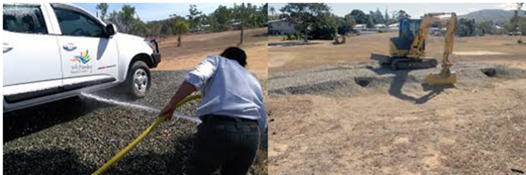
Figure 2: Collinsville Manual Washdown Facility
