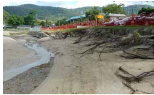
Figure 35c: Cannonvale Beach coastal erosion
