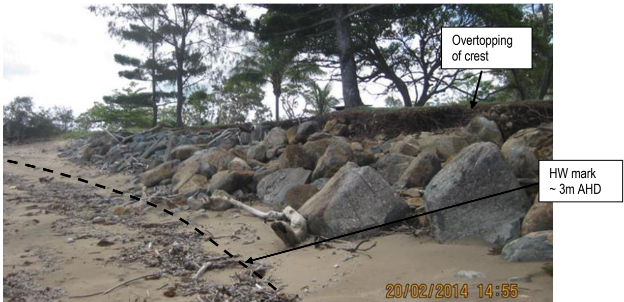
Figure 11: Seawall after Cyclone Dylan
