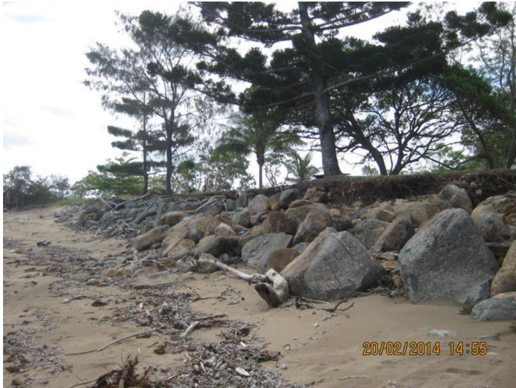
Figure 17: Present boulder wall at Wilsons Beach (overtopping damage evident)
