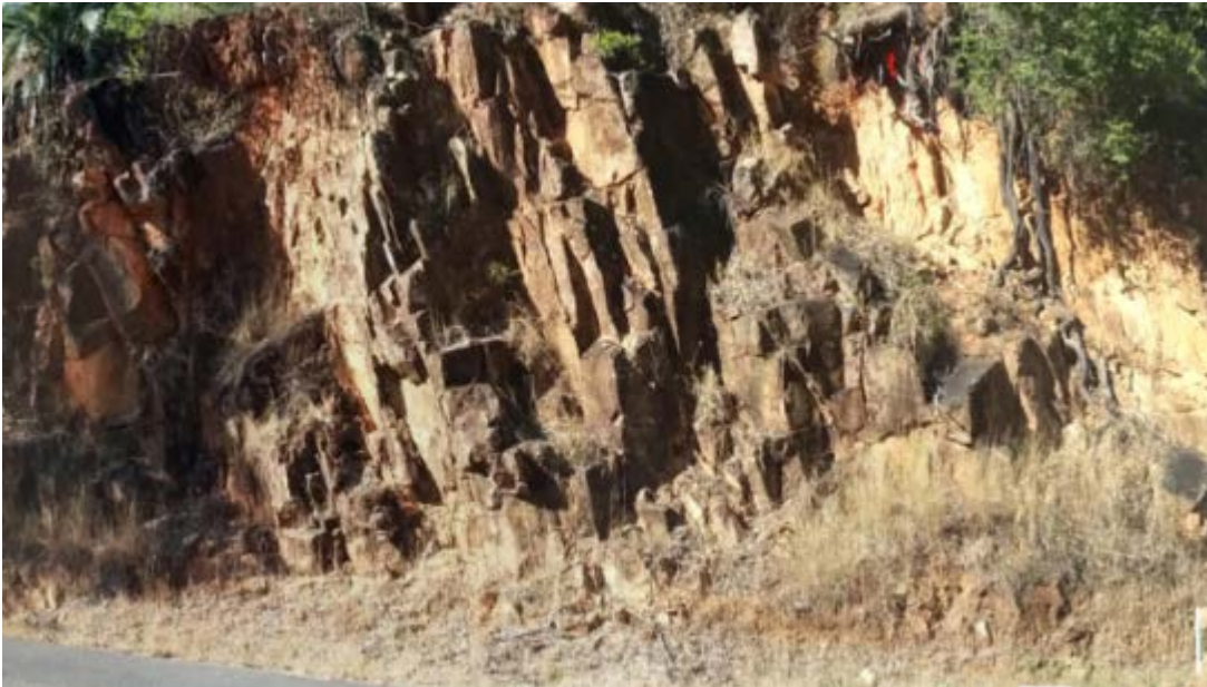
Figure 5-2 Adverse dip and jointing in a rock cutting promoting the formation of toppling failure
