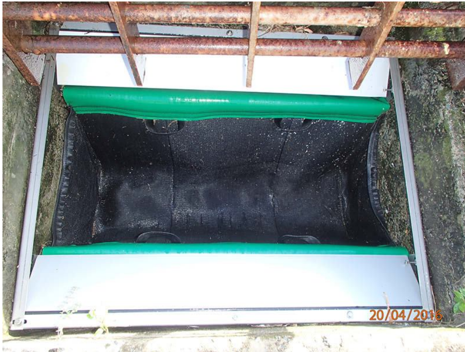
Figure 43: A stormwater inlet with a gully basket
