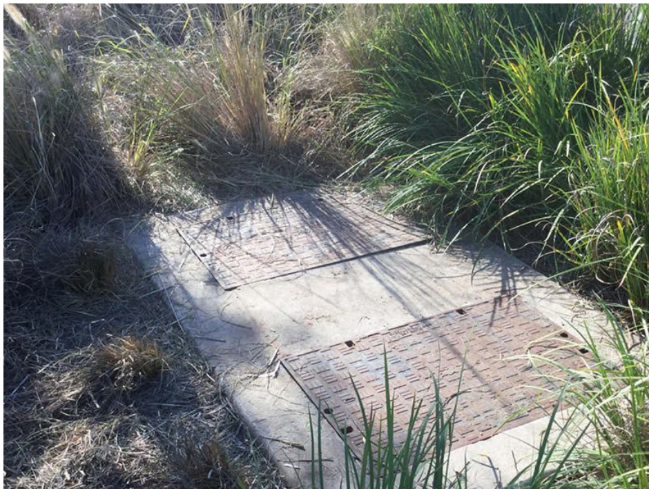
Figure 42: Example of a gross pollutant trap
