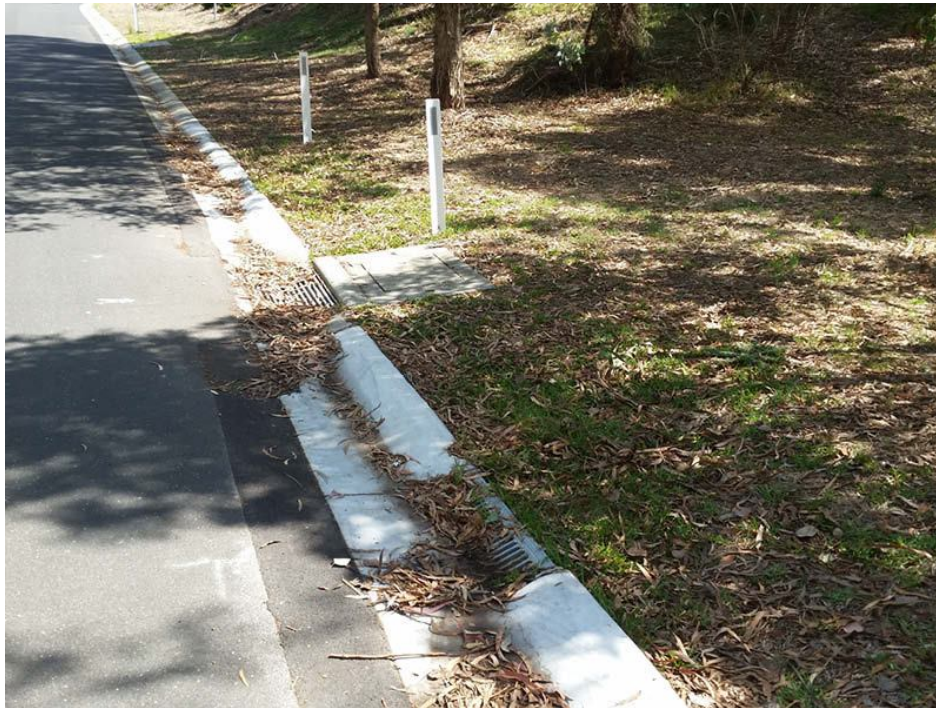
Figure 22: A turfed streetscape bioretention system in the verge
