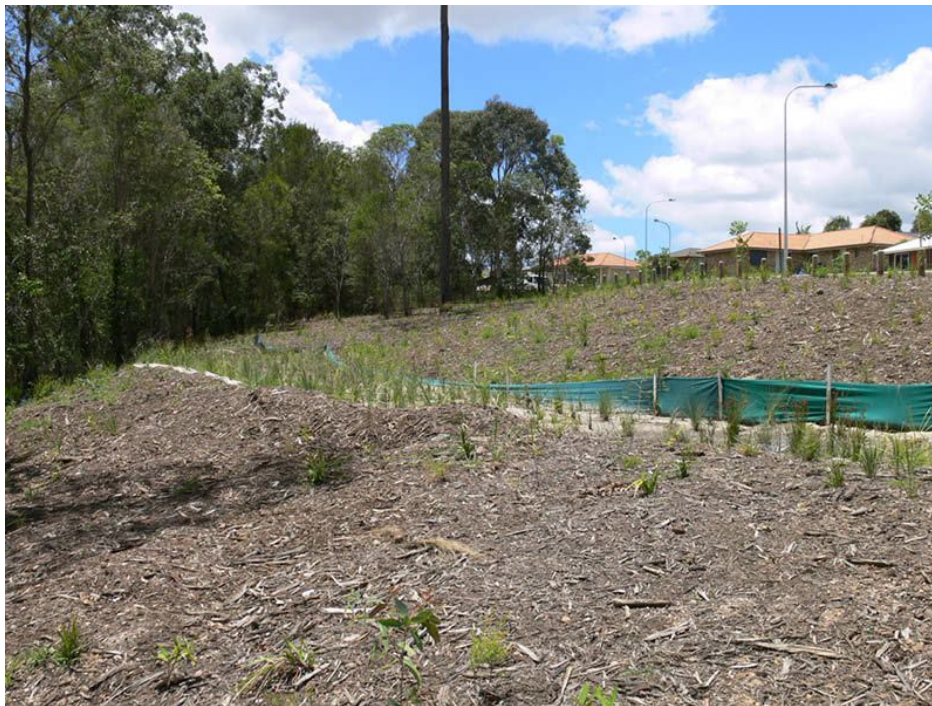
Figure 17: A newly planted bioretention system. A large batter exists to the rear right of the system. A small bund exists to the near front of the system.
