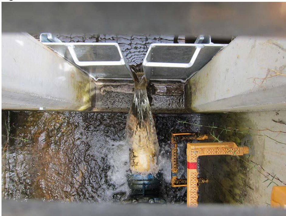
Figure 31: The outlet from a stormwater treatment wetland the day after rain
