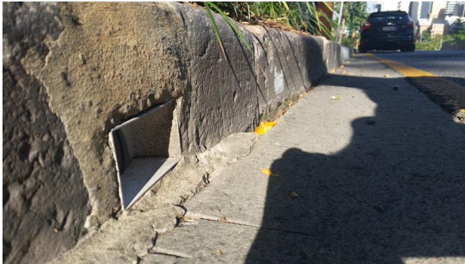
Figure 38: Pipe connection for a self-watering street tree
