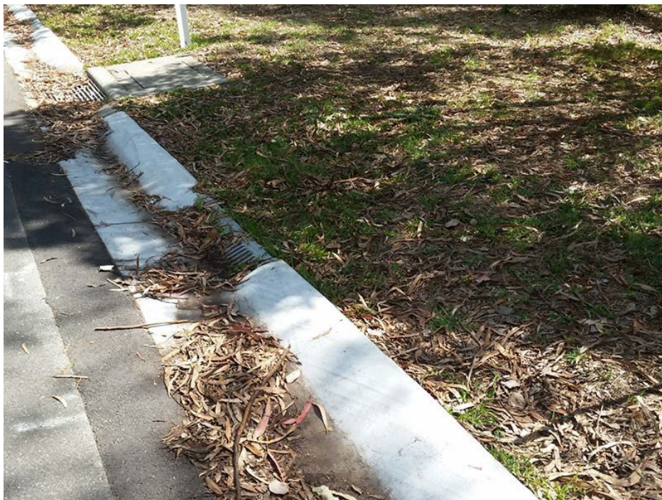
Figure 24: Example of a low tech grass bioretention system
