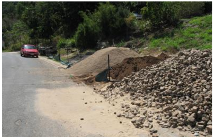
Poor site planning – stockpiles on top of the sedimen
