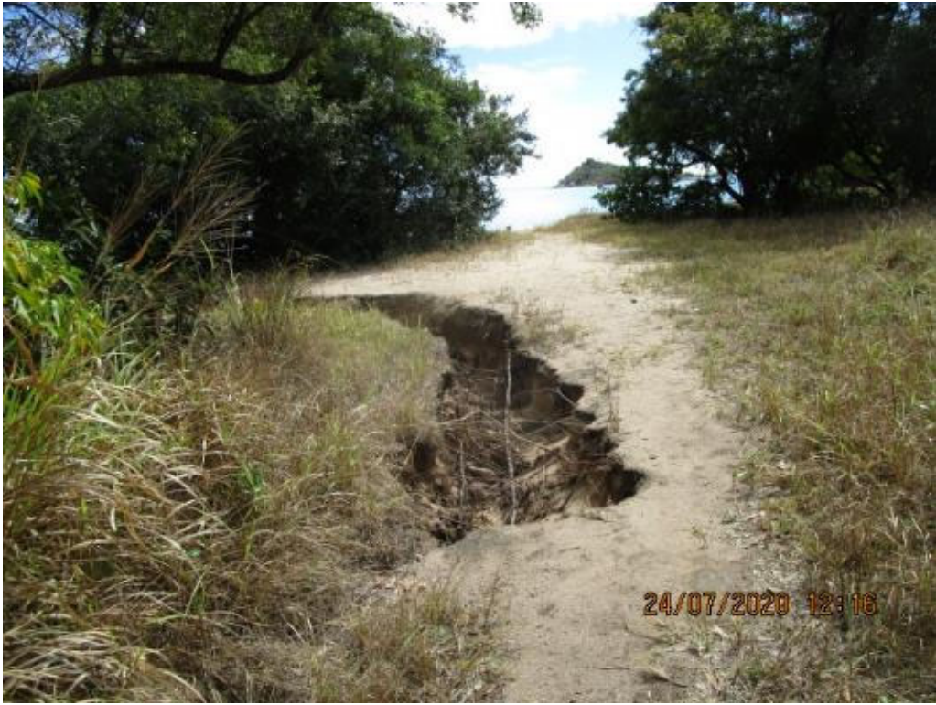
Photo 4: Erosion at Beach 3
