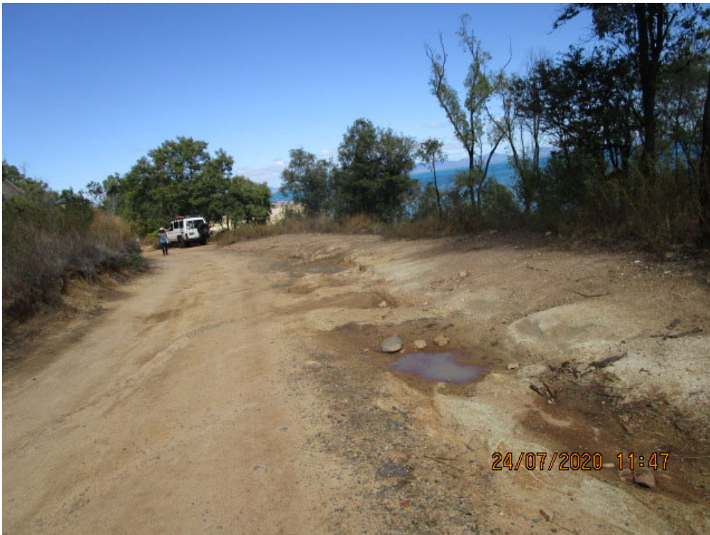
Figure 8: Erosion Caused by Vehicle Access to the Beach
